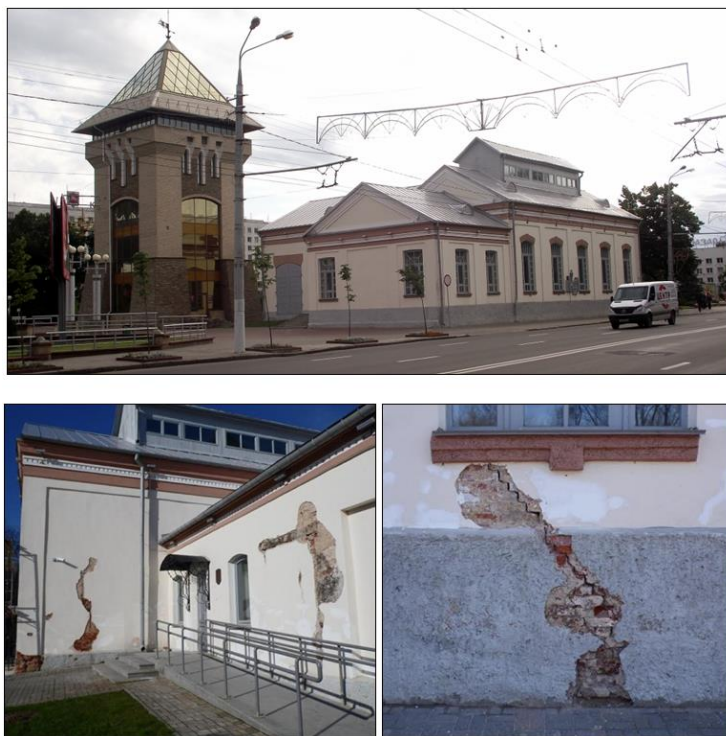
Fig. 7. Building of the first power station in Vitebsk (1897–1898) along Frunze Avenue in the historic part of the city and cracks in wall structures resulting from vibrations during the movement of urban transport (2016) [25]
