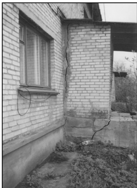
Fig. 9. Cracking in a residential building on the Lenin street, 101 in Liozno (Vitebsk region) as a result of heaving of moraine soils (2005) [10]
